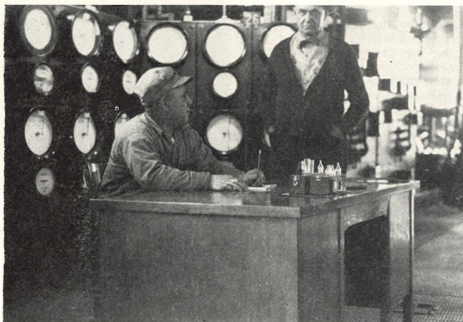
Control Panel at Cooling Water Pump House No. 2. Everett Harrington, cooling water shift foreman (seated), and F. J. Schinagle, cooling water general foreman (standing).
