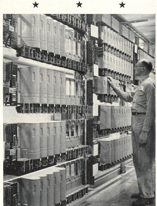
HAROLD NELSON, Shell's telephone man, checks a line-finder mechanism in a bank of new equipment in the basement of the Control Laboratory. As a result of the new equipment, additional lines can be added to the Shell system.
