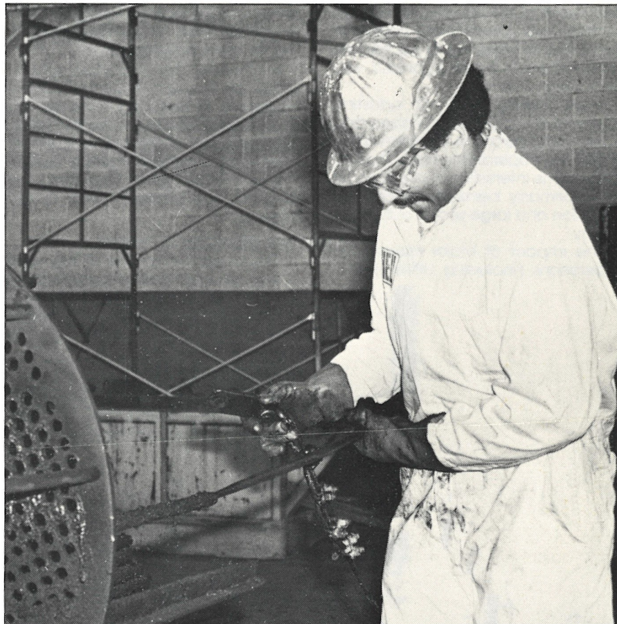
Removing tubes from a Visbreaker Flasher heat exchanger to make way for new ones is Jesse Rockingham, boilermaker. The task is part of Major Projects, a three-year yield improvement, modernization and energy conservation program at Wood River.
