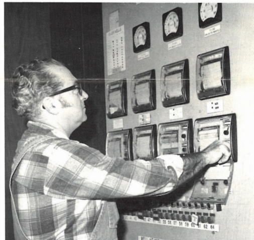
WATER ADJUSTMENT. Ernie Johnson, operator-1, makes an adjustment to the level of a fire water storage tank from the Utilities Control Center (UCC). The UCC is the central control point in Utilities.
