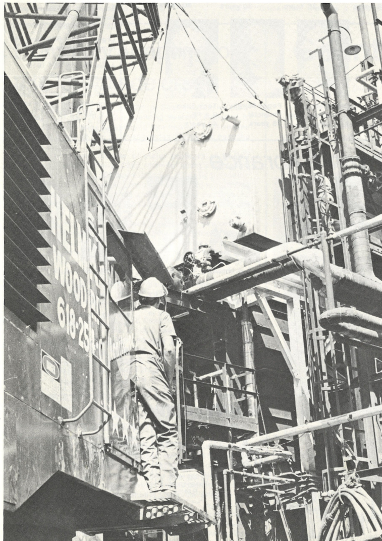
The unassuming gray box being put into place on Boiler 15 can save the Complex close to $600,000 a year in fuel costs.
