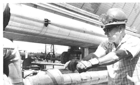
DESALTING of crude to reduce corrosion in downstream units is an early step in the distilling process. Operator Carl Lorenz opens a valve at the electric desalter.
