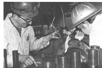
CAREFUL CHECK. Machinists Tony Morris (left) and Arnie Henke caliper mechanical equipment at the Wet Gas Compressor No. 2.
