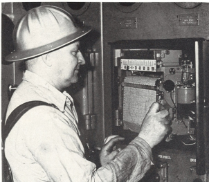
E. P. Liesmann, senior instrument man at the Lube De-Asphalting and De-Waxing plant, is adjusting a Brown multi-point temperature recorder located in the plant's control room. Instruments not only record temperature but can also control, indicate, and measure. This particular instrument shows temperature variations, and operators need it to run their units efficiently.
