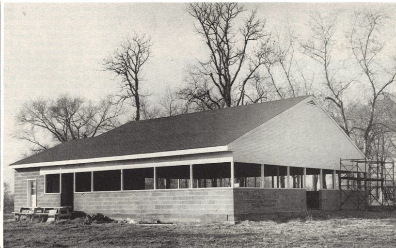
One of the major activities of the SRA is the Kendall Hill project. The Shelter has been a big job for SRA members, and has been constructed by volunteer labor, with the exception of pouring the concrete floor. The building is expected to be completed this summer. Kendall Hill also includes a lighted softball diamond, picnic area, and playground equipment.
