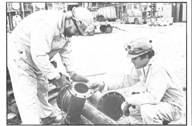
Below: Inspectors Bill Jacobs and Ron Baggett examine the gasket surfaces of new pipes for Cat Cracker-2.
