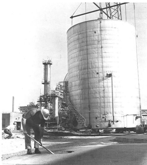
As the tank moves forward, yardman Dick Hilyard clears a spot on the new foundation where the tank's water trap will fit.
