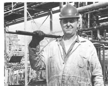
JIM AKERS , pipefitter 1st. "Are these pipes heavy? Naw, I just carry them on my right shoulder to balance the chew can in my left pocket."
