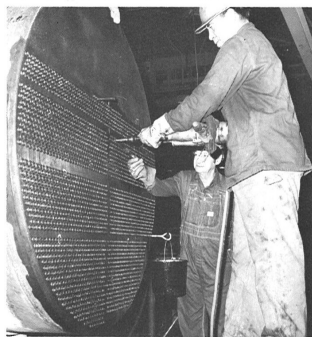
"Rolling the tubes." Using a special tool, Frank Carrigan expands the outer couple inches of each tube to assure a tight fit. Leon Little applies oil to reduce friction. Both are boilermakers.
