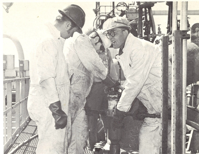
The final steps of a shutdown. In this case at the CR-3. While Don Perdun, boilermaker helper, looks on, Harry Kulp, boilermaker helper, and Dick Milcic, boilermaker 1st, use an impact wrench to head up a reactor.
