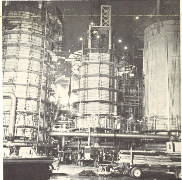
A nighttime view of the refinery in March, 1971. About 80 people a day, including men from virtually all crafts, worked night and day on two shifts through the weekends on a shutdown of catalytic reformer no. 3 in the Aromatics department.
