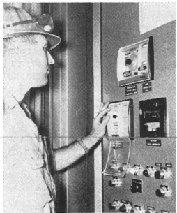
ADJUSTING CONTROLS on the console of the new asphalt blender in the Lubricating Oils Department is Operator 1st Adolph W. Borgini. The new equipment blends materials as they or being loaded in railroad tank cars or trucks.
