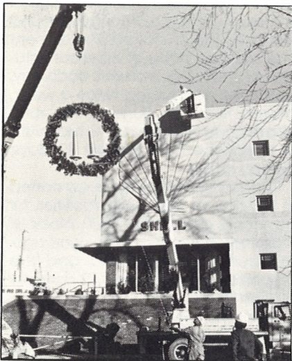
Workers prepare to attach a large Christmas wreath to the side of the Main Office Building. Once again, the Complex is decked out in Christmas lights, ornaments, trees and other decorations.
