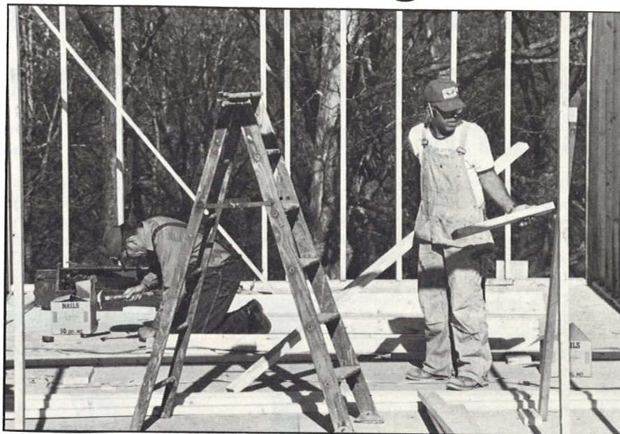
Working on the Teen Challenge building project are Harry Woods (left) and Tom Schilling. The new facility will contain a dining room, offices and classrooms for the staff and residents. Teen Challenge is a rehabilitative center in High Ridge, Mo.
