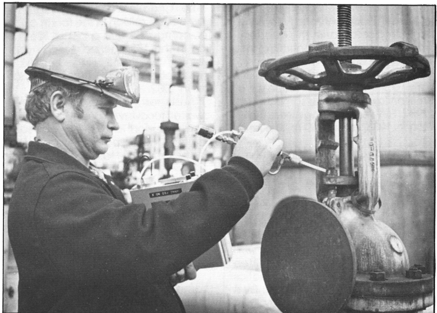
Paul Sibley, operator at Aromatics East, uses a detection instrument to test a CR-3 valve for vapor leakage. Approximately 31,000 Complex valves, pumps, compressors and process drains are regularly monitored for liquid and vapor emissions; those that leak are repaired.
