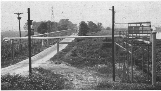
SHELL'S NEW ASPHALT LINE to the barge loading docks on the Mississippi River is shown here where it comes from beneath the levee and runs west toward the river. The pipeline, according to Union Electric Co. is the longest electrically heated pipeline in the U.S.
