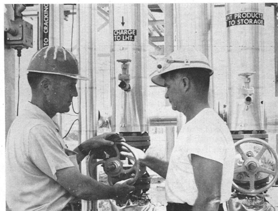
OPENING THE VALVE to put charge stock into the Refinery's new Lube Oil Hydrotreater is Operator 1st Victor P. Buese. Watching the operation which brought the new unit on stream is R. A. Jones
